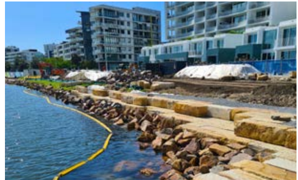
Beginning works on Honeysuckle Park, a $4.2-million public space for the entire community in the Newcastle CBD
