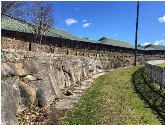
Figure 6: Exposed sandstone associated with grading to create a sports field, facing northwest
