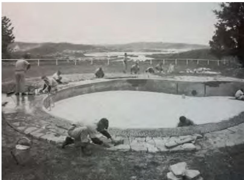
Figure 21: Boys at work on the construction of the children's swimming pool, 1968 (Image DCS/DJJ HC)
