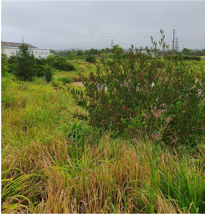
Plate 3 - Road widening works encroaching on fringe vegetation of the existing detention basin
